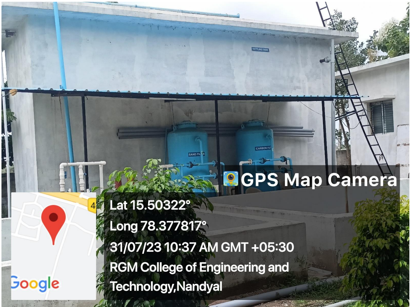
Waste Water Recycling /Management System
