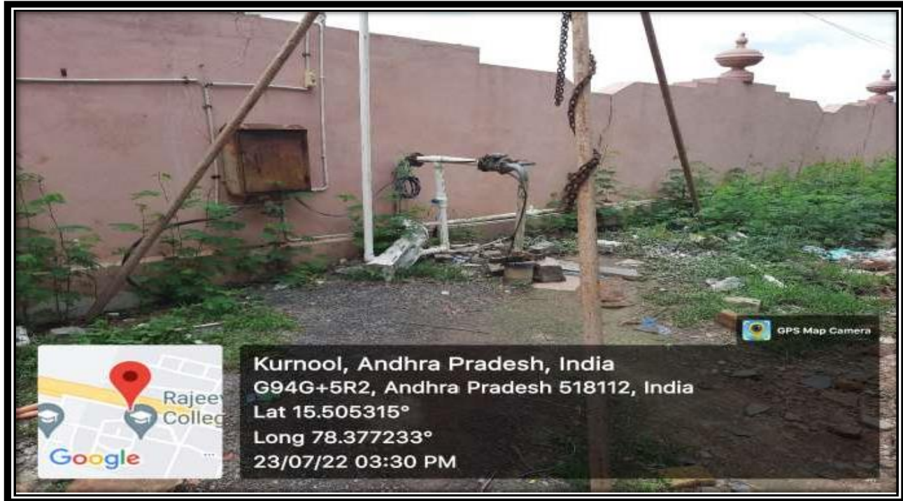
Bore well near the Main Gate
