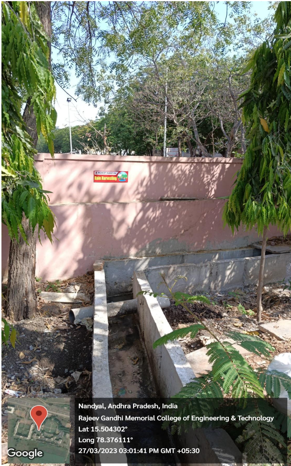
Rain Water Harvesting System
