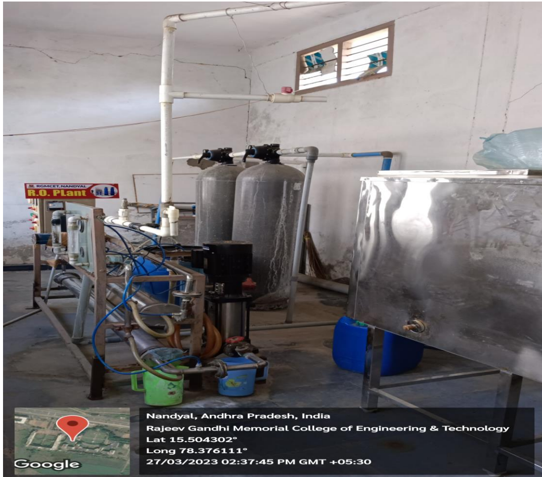
R O Water Plant in the Campus
