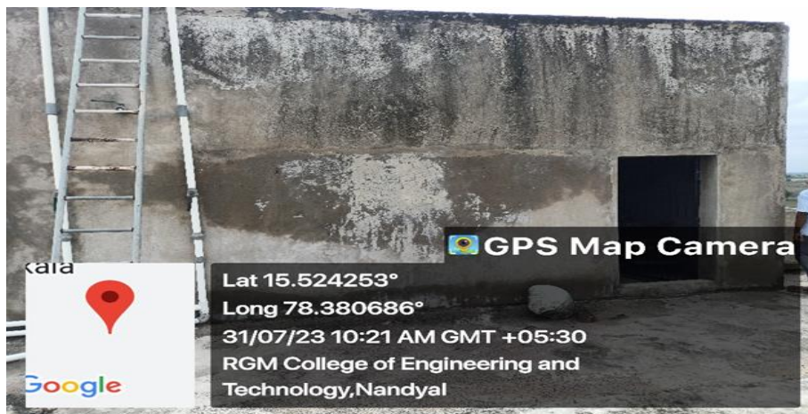
Water Tank on the top of ME Block
