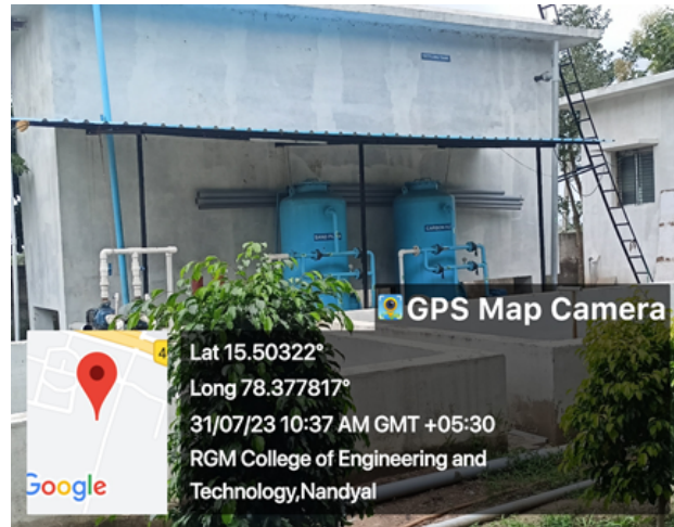
Waste Water Recycling Plant in front of ME Block
