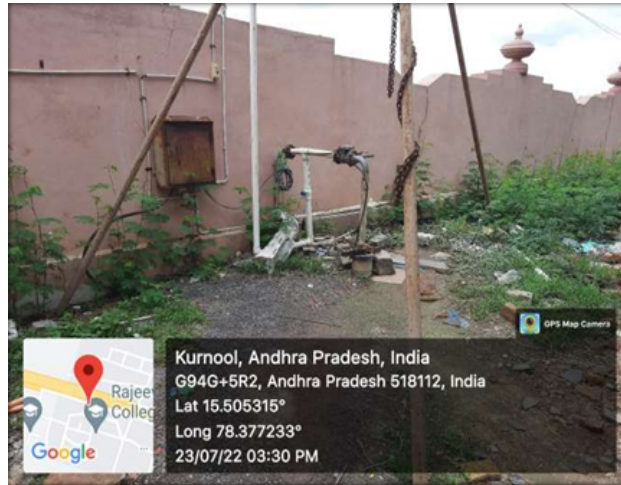
Bore well near the Main Gate
