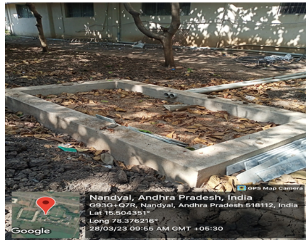
Rain Water Harvesting Unit near the Canteen
