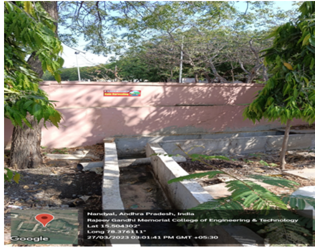
Rain Water Harvesting System
