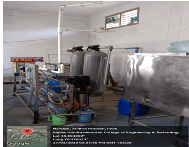
RO Water Plant in the Camp
