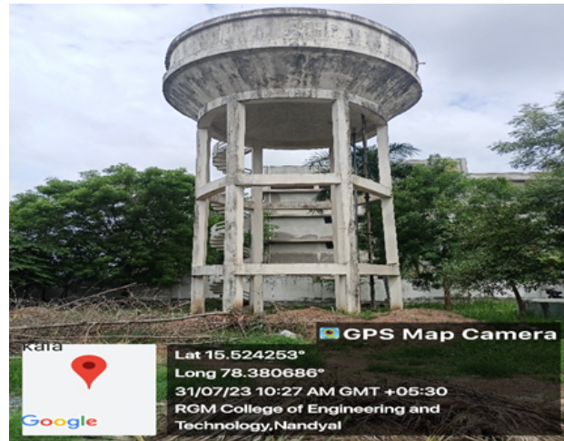
Overhead Tank in front of CE Block
