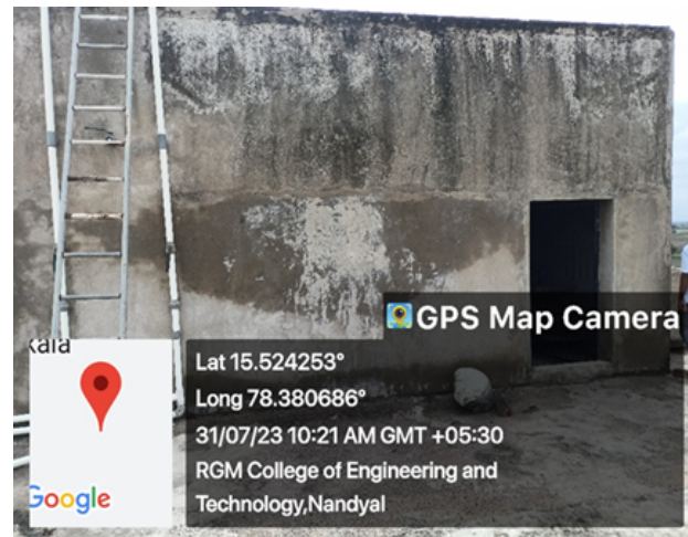
Water Tank on the top of ME Block
