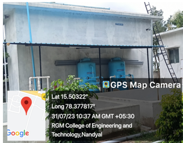
Waste Water recycling System
